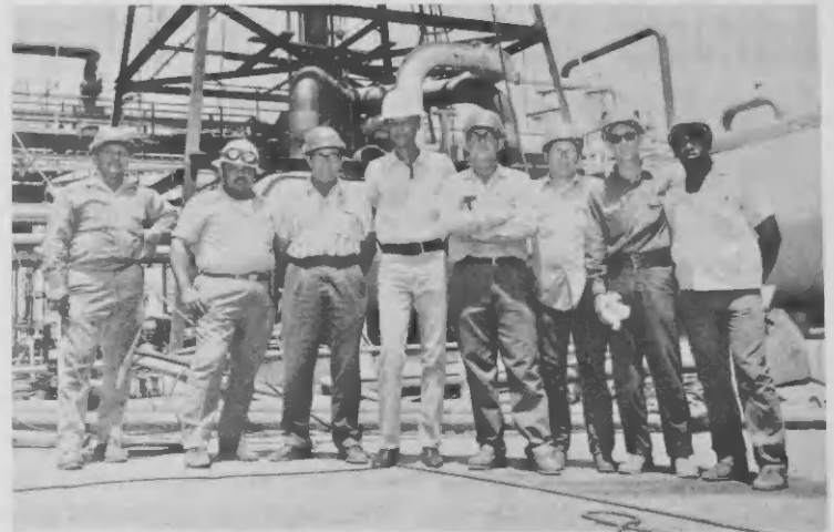
The keymen in the hoisting of the new smokeless tip: (from l to r): Gene Dean, CB&I high rigger; Gilberto Maduro, Lago Field engineer; Irving J. Estelle, CB&I local superintendent; Errol J. Bardouille, Project Leader; William Burkeen, CB&I superintendent, Thomas Gardner, Carl McKay, CB&I high riggers; and Teodor Patterson, CB&I hoist operator.
